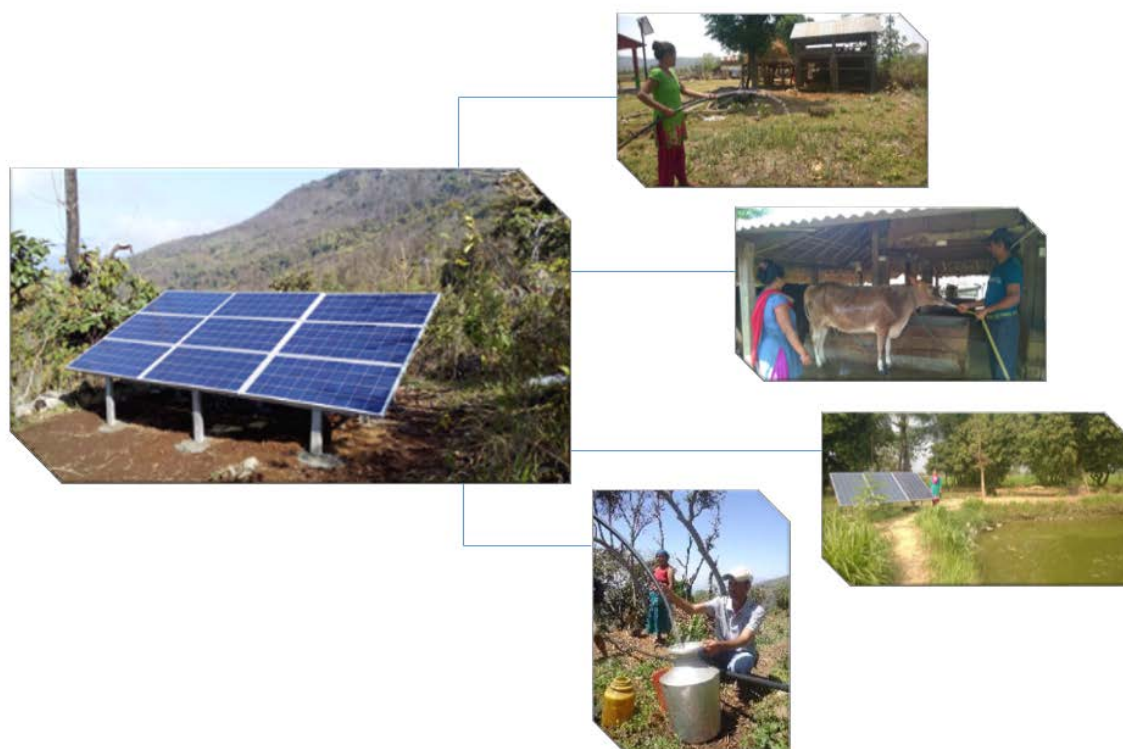
Figure 1: Photovoltaic water pumping used for irrigation, livestock watering, fish farm and drinking water
