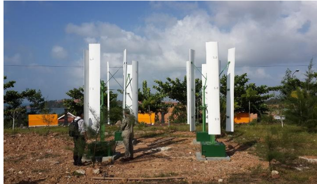
Figure 10. Vertical Axis Wind Turbine 2 kW
