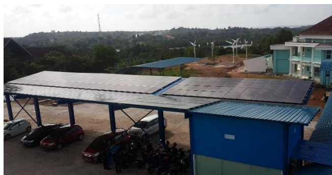
Figure 7. Solar Module Carport in UMRAH
